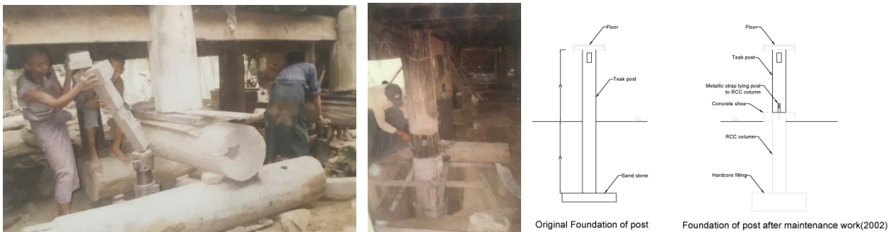
Fig. 5 Lift wooden post with jack, connection between wooden post and RCC column and types of post foundation. Source: The first two photographs are taken by Department of Archaeology and Museum, 2002 and the last one is drawn by author, 2022.
