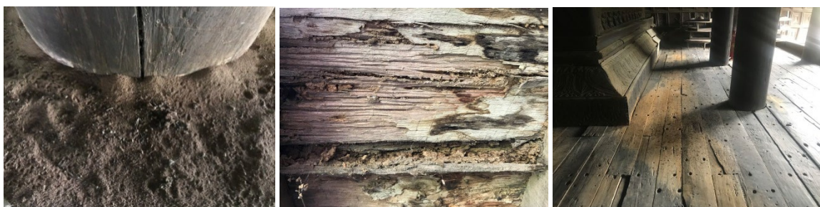
Fig. 8 Damage of wooden post, veranda floor and interior floor caused by animals. Source: Photo by author, 2022.
