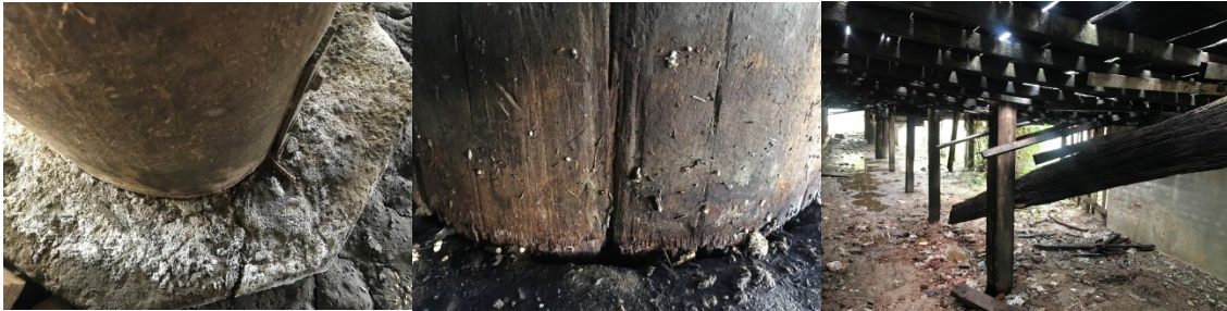
Fig. 7 Fungi on concrete shoe and wooden post, and the condition of main beam under the veranda floor. Source: Photo by author, 2022.
